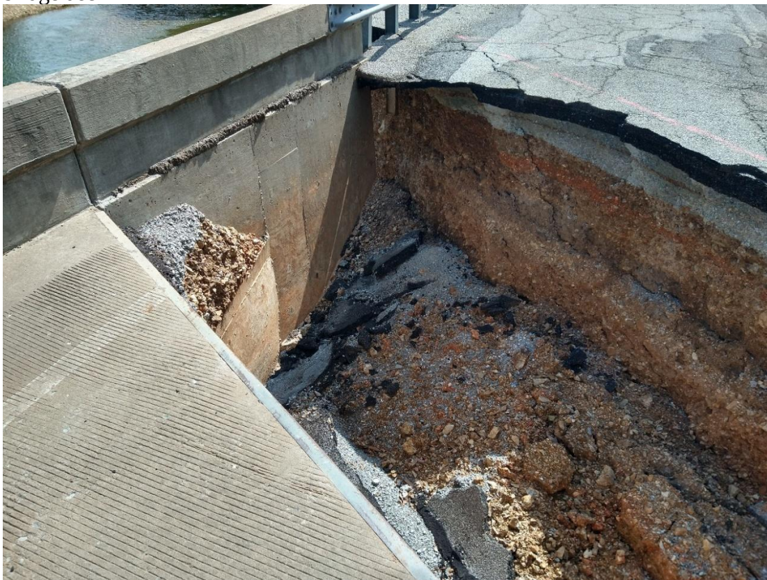
Picture #2 - East bridge approach looking at washed out material beneath wing wall from bridge deck
